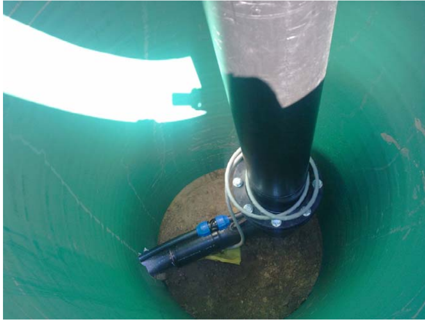
Put mixt biogaz/levigat – detaliu cu tevi transport biogaz si levigat
