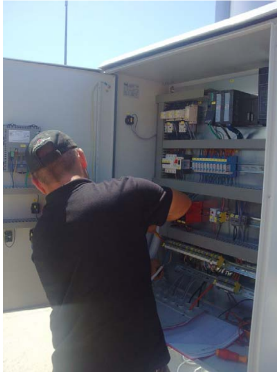
Firida container regularizare debit biogaz
